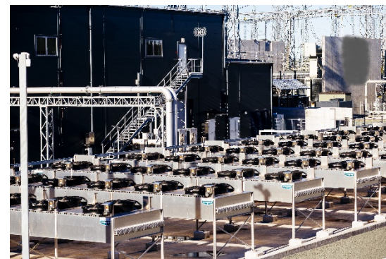
Plate 5.23 – Typical Outdoor Heat exchangers Image: ©GE
