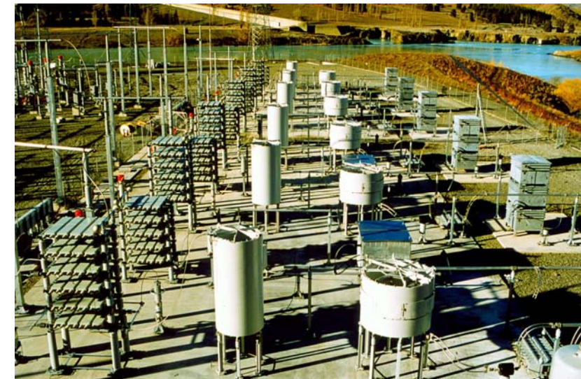
Plate 5.11 – Typical AC Switchyard Harmonic Filters Image: ©ABB
