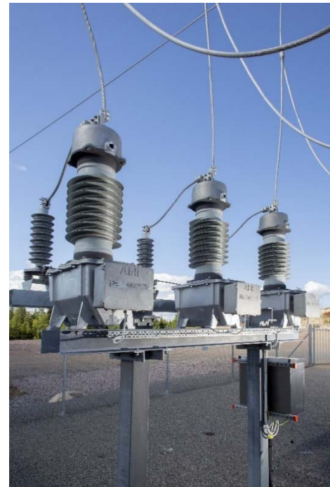
Plate 5.16 - Typical Voltage Transformer Image: ©ABB
