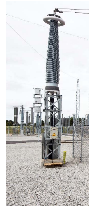
Plate 5.6 – Typical 400kV Cable Terminations Image: ©GE
