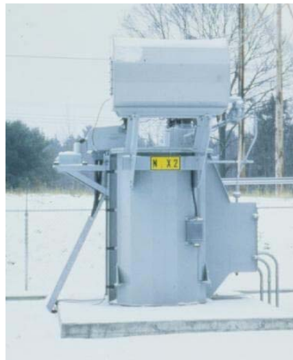
Plate 5.12 – Typical Auxiliary Power System Image: ©ABB
