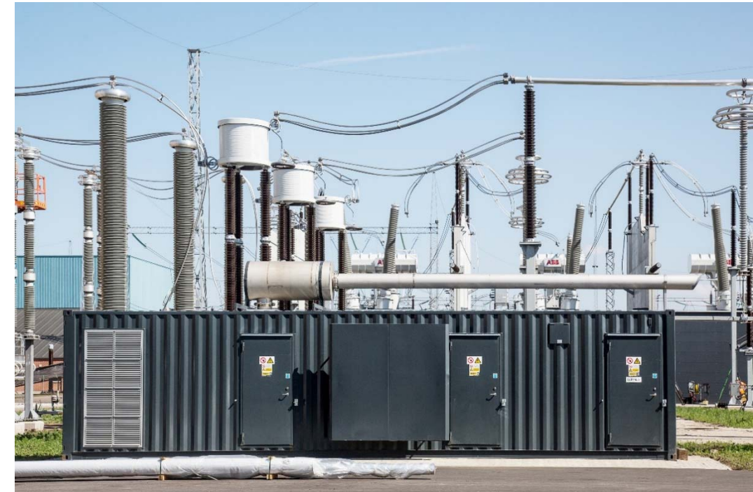
Plate 5.13 – Typical Diesel Generator Image: ©ABB
