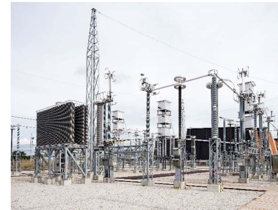
Plate 5.8 – Typical Lightning Masts Image: ©GE
