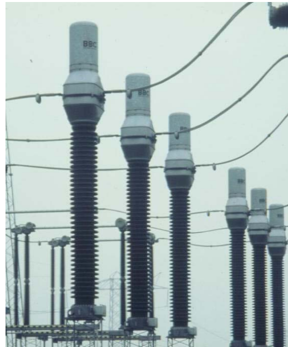
Plate 5.15 – Typical Current Transformer Image: ©ABB
